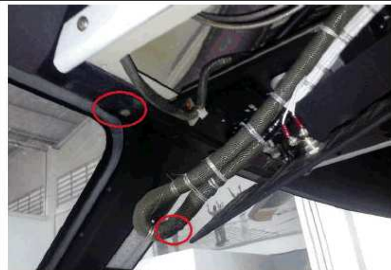
Bolt head location and wiring burn
